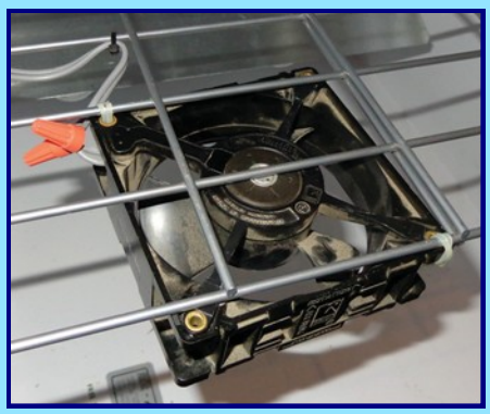
A fan is mounted underneath the wire shelf.
